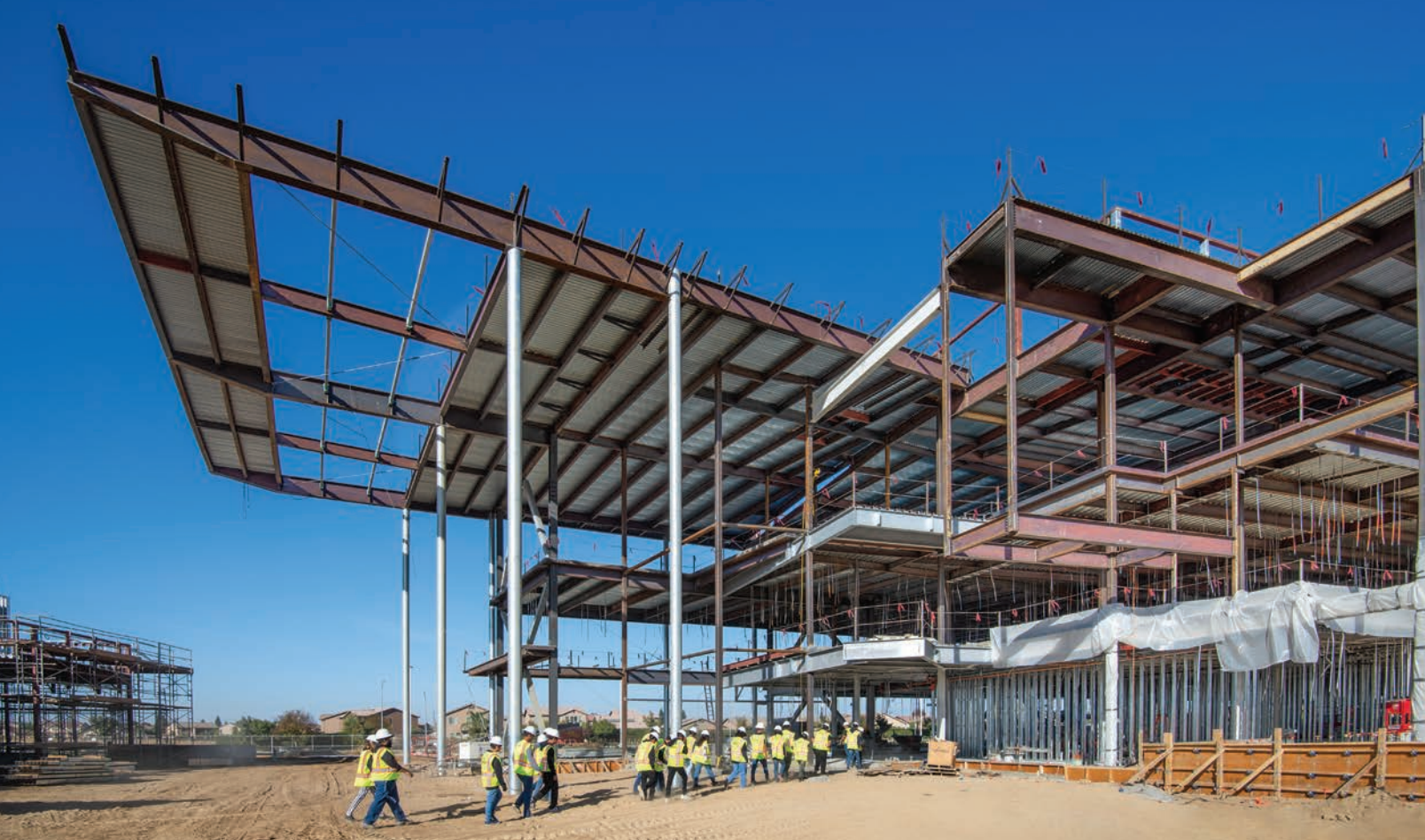
Valley ROP Students tour Phase II of the Sanger Education Complex being built by Harris Construction. The initial new High School buildings will be open in late 2023.
