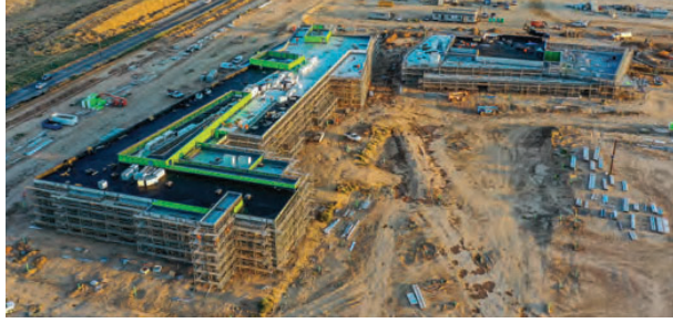
Project by Harris Construction: Sanger Ed Center (Sanger Unified School District). Photo during construction of Phase 1, a 124,404 sq. ft. middle school complex. The project is now in Phase 2, a 125,290 sq. ft. high school project.
