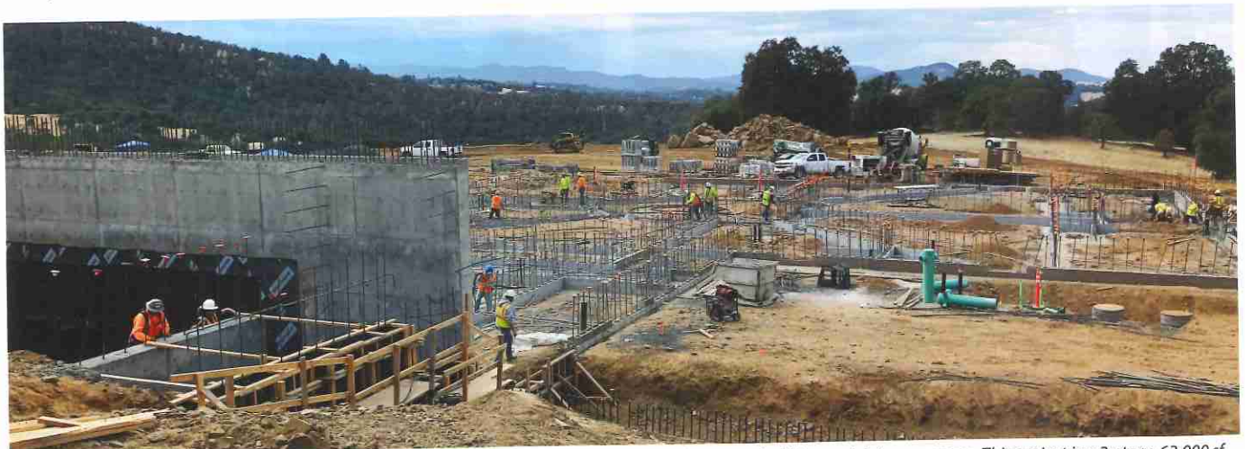
Harris Construction also specializes in building food- and dairy-processing plants, hospitals, private facilities, and civic campuses. This project is a 2-story, 63,000 sq. ft. detention center being built in Sonora, CA. Senior Project Manager, Geno James, is leading the team on this Harris project.
