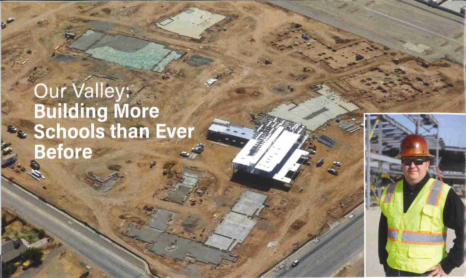
Aerial View of Madera Unified School District's newest school project: Matilda Torres High School. The 277,000 sq. ft campus over 55 acres will be completed in late 2020. This will be the third high school for MUSD in Madera, CA. Inset photo: Assistant Project Manager, Stephen Hamett, with Harris Construction - standing in front of some of the first steel to go up on the Matilda Torres High School project.
